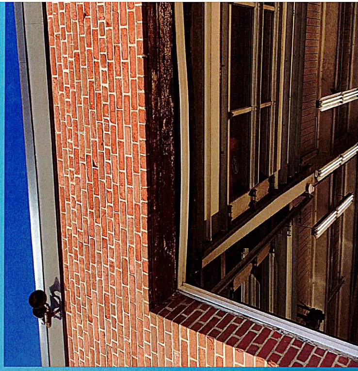
Frames are bent
