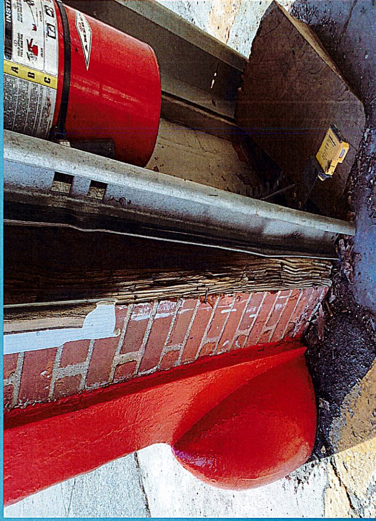
Rotted wood on doors
